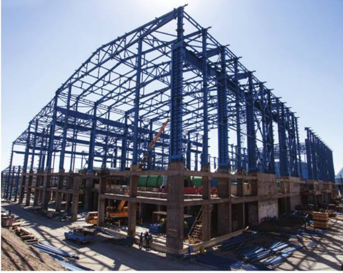
● The main hall of Concentrate Unit- Sangon site
