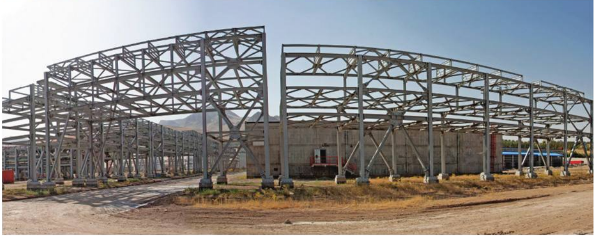
● The steel structure of petrochemical plant of Kermanshah- unit of Urea and Ammonia
